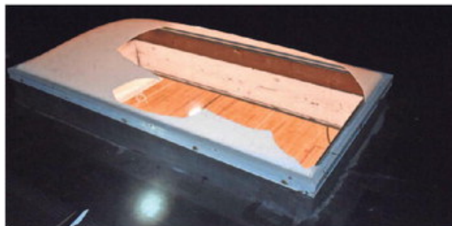
A skylight where an 18-year-old Penfield student fell through the roof at Bay Trail Middle School early Thursday. PROVIDED
